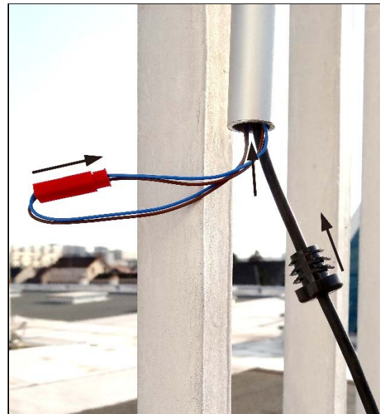
Figure 2–6 – Powering on the anemometer
